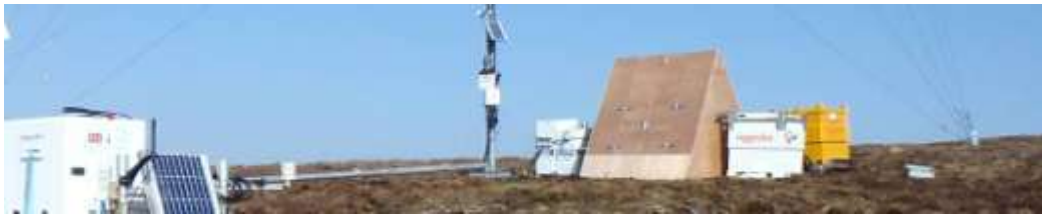
Figure 7.3.3: 'Tent' with ventilation covering generator
