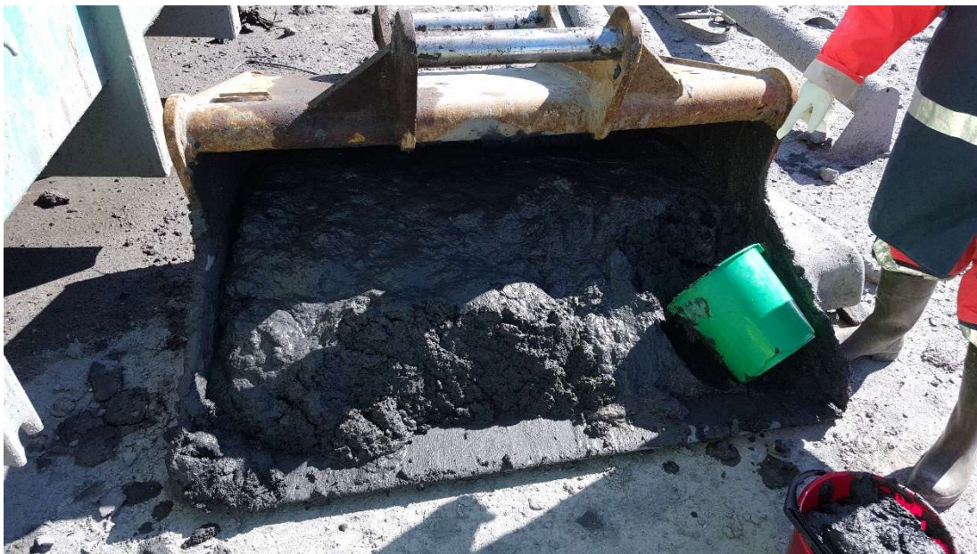
Figure 1. Dredging and sampling of organotin and metal contaminated sediment from Arendalshamnen in Gothenburg, Sweden. Photo: Anna Norén
